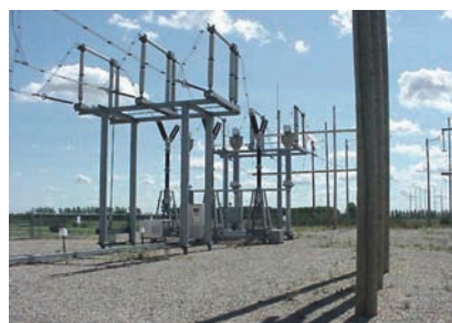
Fig. 8. Case 4 Live Tank Circuit Breaker
